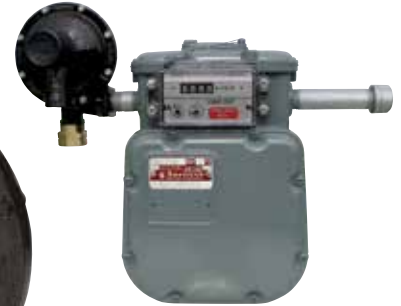
Attached to Vapor Meter
